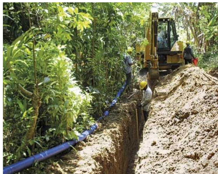
More than 200 000 electrofusion fittings of the ELGEF system are installed in Ampara
